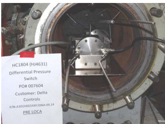
Delta Switches mounted in LOCA chamber
